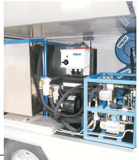
WHU water heater along with other DYNASET high pressure equipment installed to mobile pipe cleaner.
